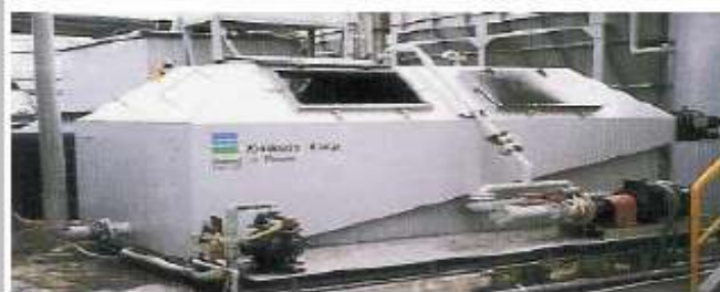
Smp-DAF in operation
