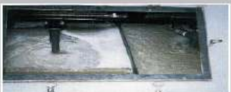
Approx. 60% of contaminants sludge area accumulated in the first cellalon e
